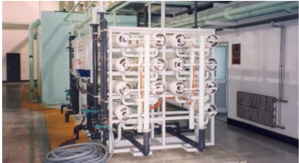
FILMTEC™ BW30-400 elements are used in the second-pass stage of the desalination process at the Huaneng Weihai Power Plant. (Photo courtesy of Huaneng Weihai Power Plant.)
