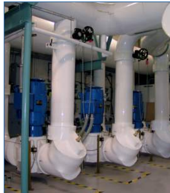
District Cooling Project, Phoenix, U.S.A.
