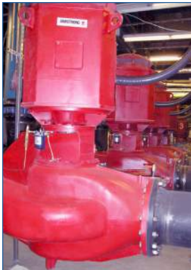
Enwave District Cooling Facility, Toronto, Canada.
